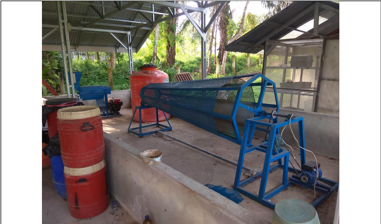
Example of Organic Waste Composting Facilities
